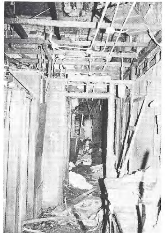
Looking north from area of origin down north-south corridor toward main corridor. Note the ceiling construction. NFPA
