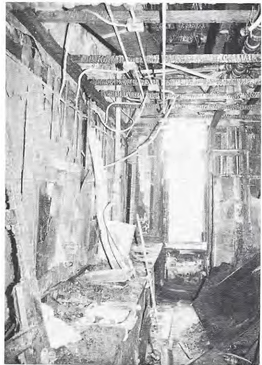
View of bathroom from north-south corridor. Area of origin is at far end of room at left of window. NFPA
