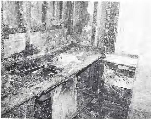
Area of fire origin in bathroom. Fire started under counter, between window and sink. NFPA
