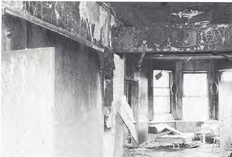
Looking west down main east-west corridor. Note damage where north-south corridor connects with the east-west corridor near left center of photo. NFPA
